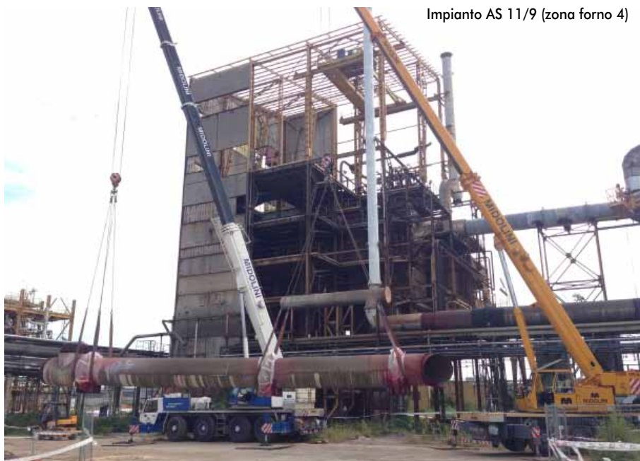
Impianto AS 11/9 (zona forno 4)
