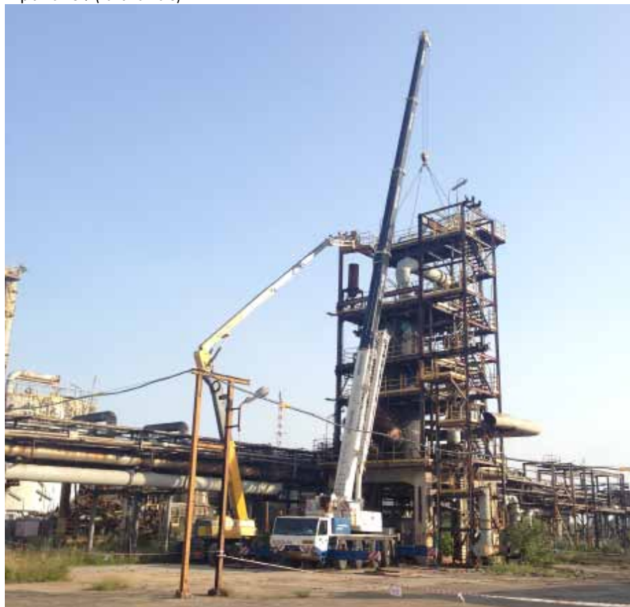
Impianto AS 9 (zona forno 6)
